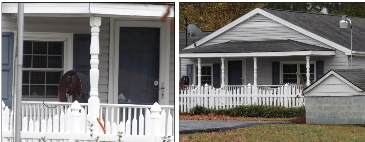
Photo 22: Turner’s Tax Service, 13392 N.C. Highway 903, Door Detail (Left) and Porch Detail (Right).
