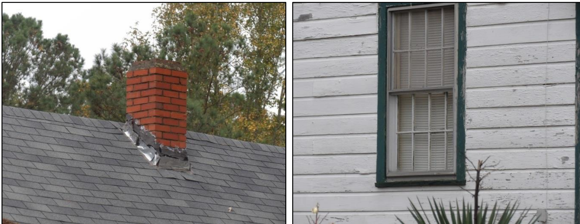
Photo 19: House, 101 Roosevelt Street, Chimney Detail (Left) and East Elevation Window Detail (Right).
